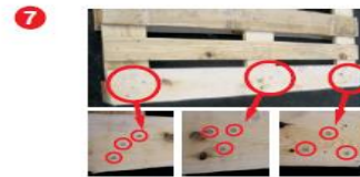
7 Unlicensed nails or irregular pattern of nailing.
